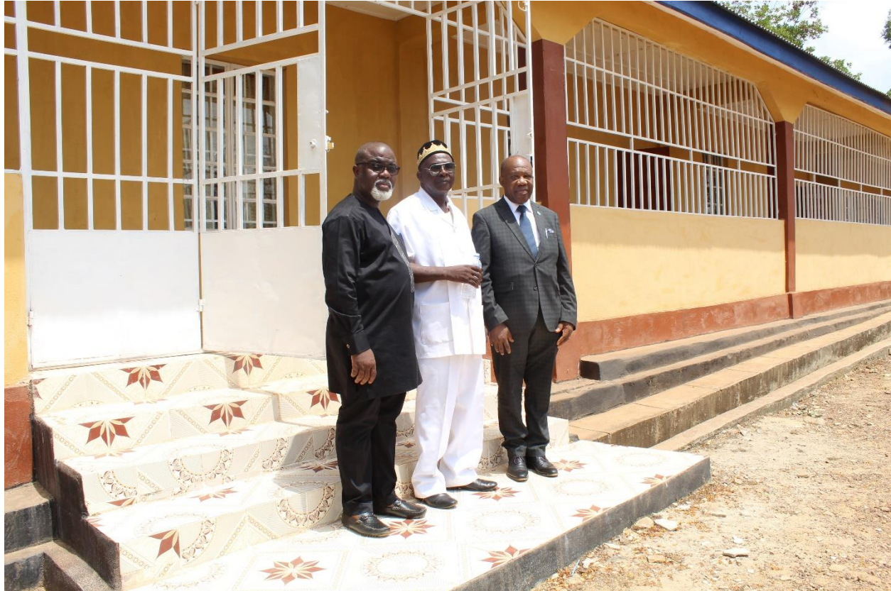
From left: National Programme Coordinator of Free Quality School Education Mr. Amara S. M. Sowa, Representative of the Council of Paramount Chiefs Frank Neekah, and MBSSE Permanent Secretary David Banya in front of the renovated building.
